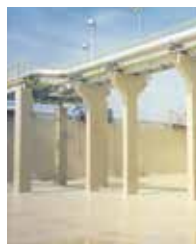
Waste Water Treatment
